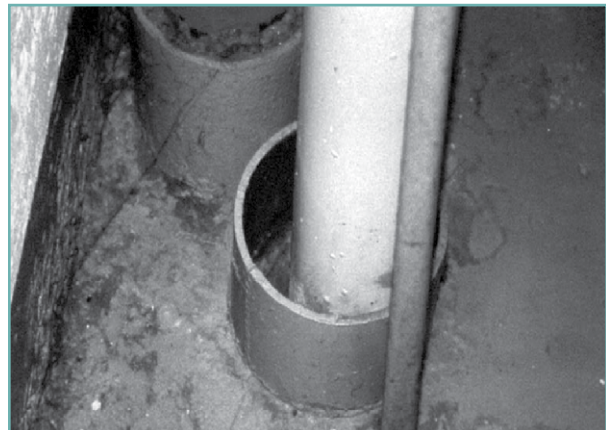
Figure 4-30 Typical conduit penetration
