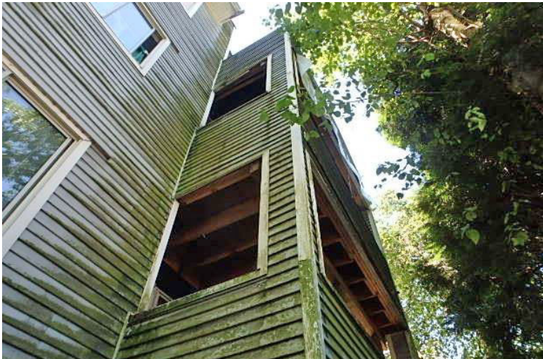
Condemned balconies: Aaron Webster Housing Co-operative
